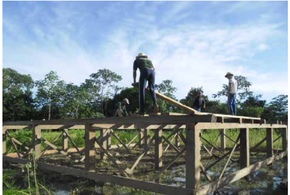
Urucurituba community: building of an elevated vegetable garden structure in Santarém, Brazil
